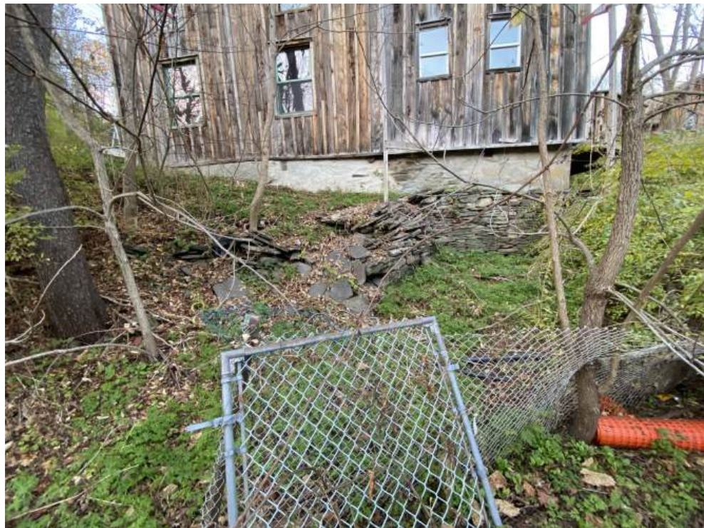
C6 L003 SITE PHOTO 5 - FAILED RETAINING WALL AND FENCING TO BE REMOVED NOT TO SCALE
